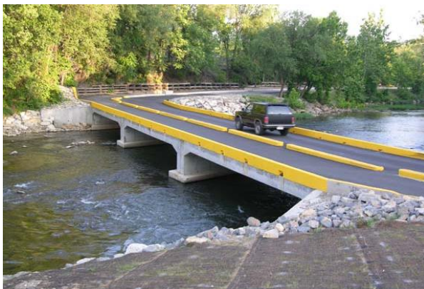
Sinking bridge on Roanoke River, NC, USA
